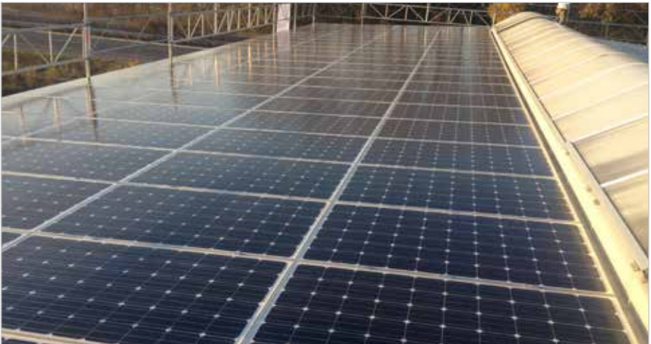
Avenches - Switzerland Installation: 50 kW | MiniRail System
