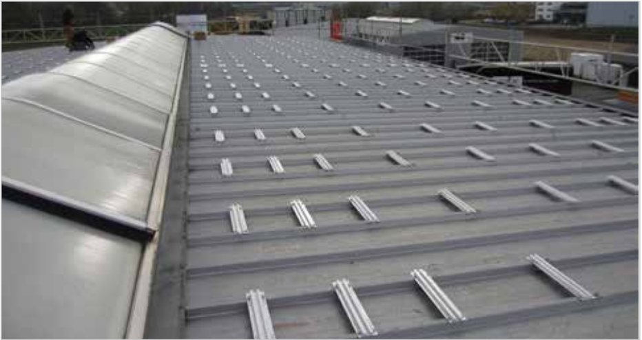
Avenches - Switzerland Installation: 50 kW | MiniRail System
